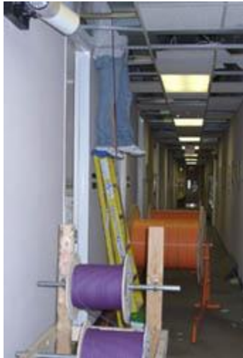
Seeing a new side of Sitterson. One of the contractors working on the network upgrade project disappears into the second floor ceiling. (Photo: Herman Towles)
